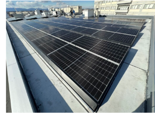
*Track record of rooftop solar panel installations for hospitals
