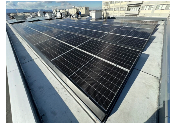
*Track record of rooftop solar panel installations for hospitals
