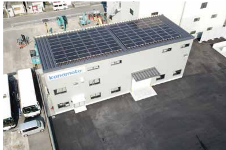
Solar Power Generation System Installed on the Roof of the Kyoto Branch Office
