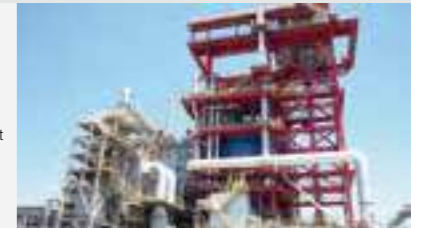
Coke dry quenching equipment (CDQ) recovers thermal energy from coke and contributes to reducing CO 2 emissions from steelworks
