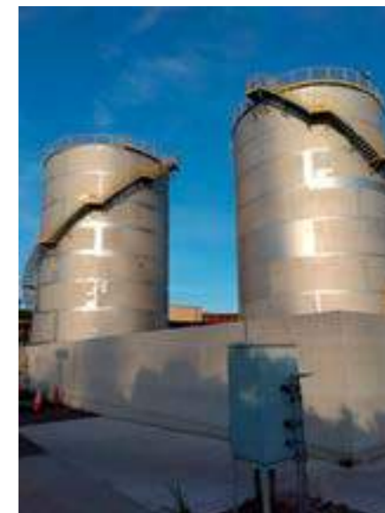
貯槽と防液堤
