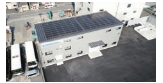
Solar Power Generation System Installed on the Roof of the Kyoto Branch Office
