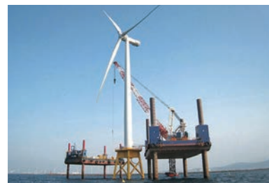
Jacketed offshore wind power generation facility under construction in Ishikari Bay, Hokkaido Photo shows demonstration facility off coast of Kitakyushu City
