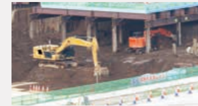
リニア中央新幹線の駅建設工事 New Station Construction for the Linear Chuo Shinkansen
